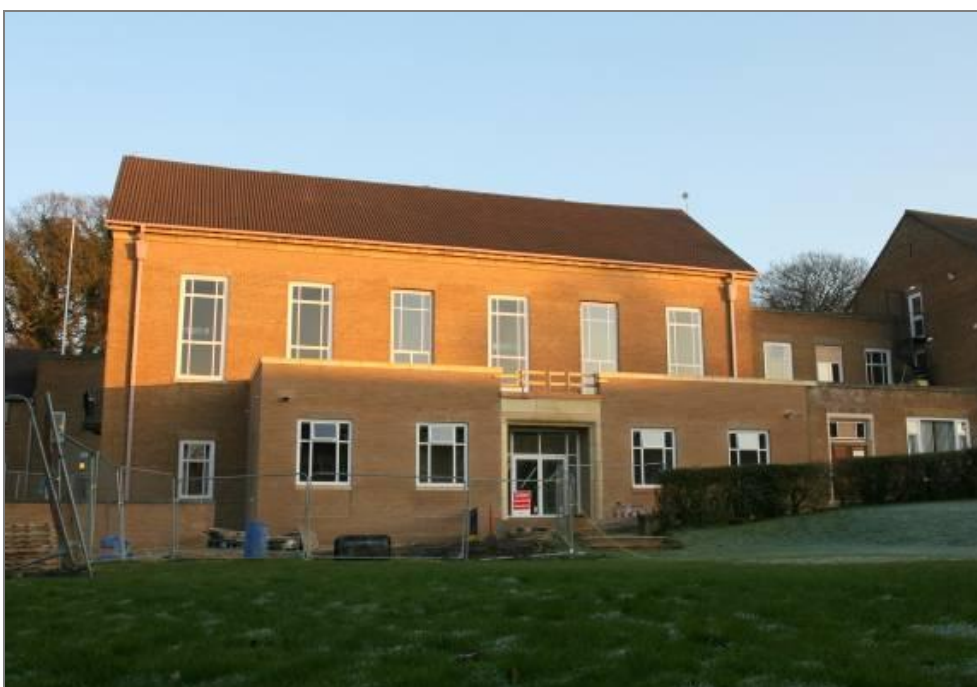
ABOVE: Front and Side View of the Development project at Grey College
